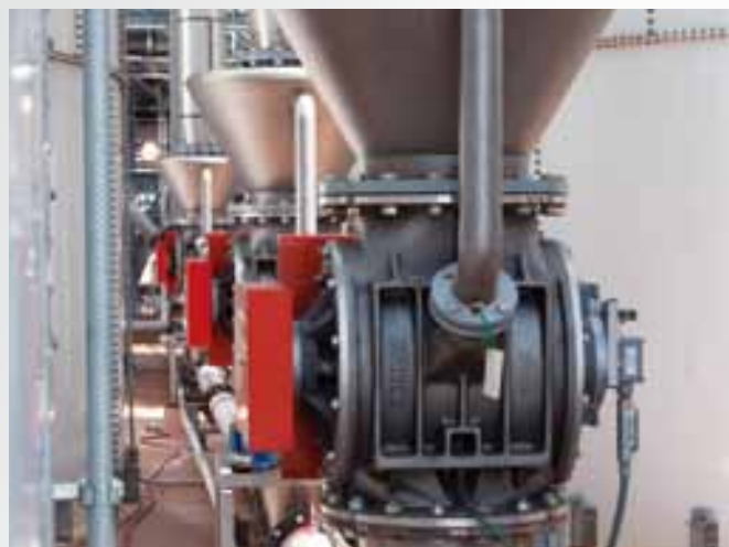
Rotary Valve Stations
