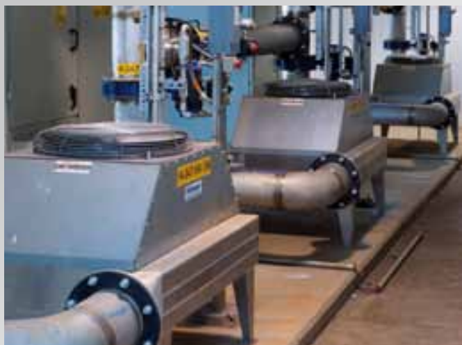
Blower Stations and Heat Exchanger
